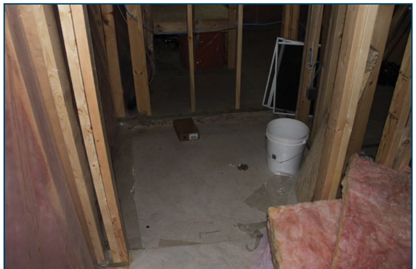
Figure 6: Elevator shaft depression in concrete floor Photo by Ron Wickman
